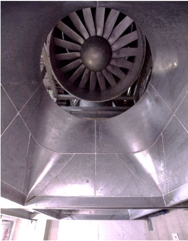
Figure 3 - Tunnel ventilation fan
